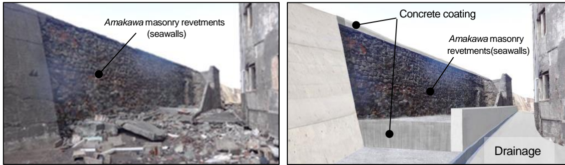
Figure 7: Images of seawall revetments conserved by Option 1 (left: before conservation; right: after conservation)
