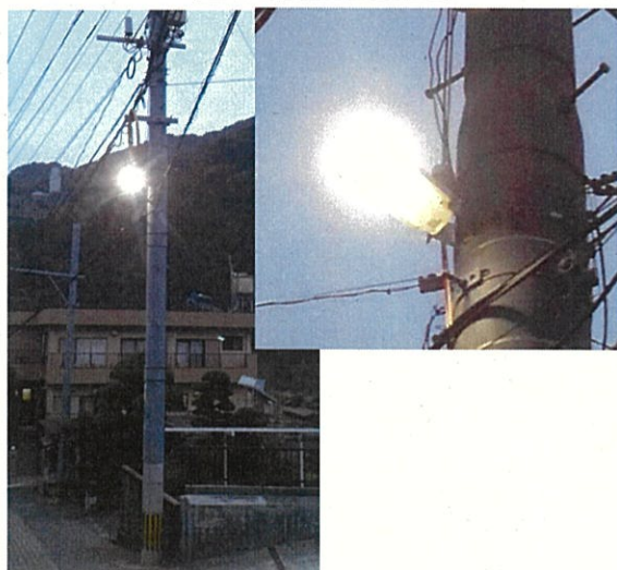
LED 街路灯 (電柱共架)
